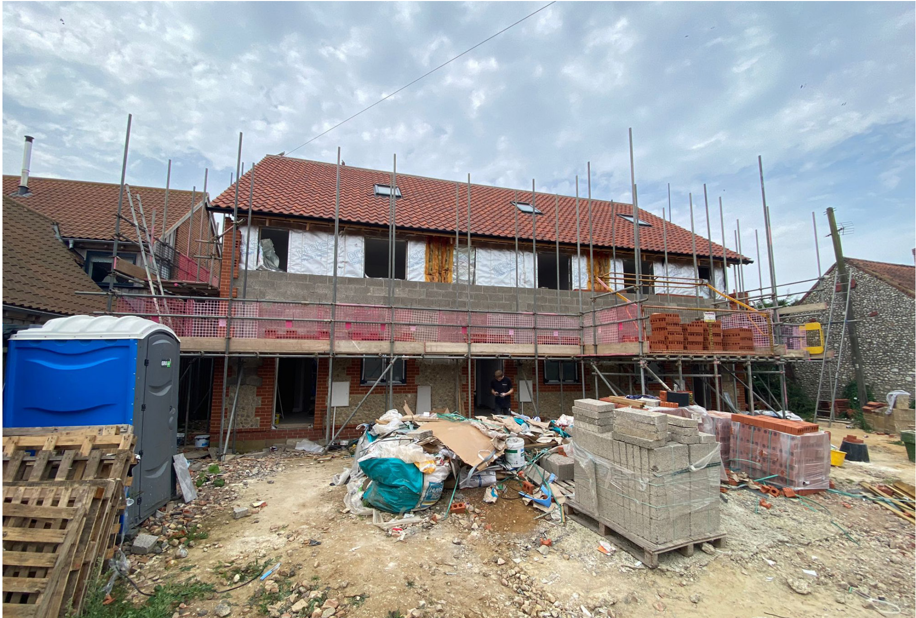
The rear of the properties are ready for the application of the cladding which is on site and ready to be applied.
