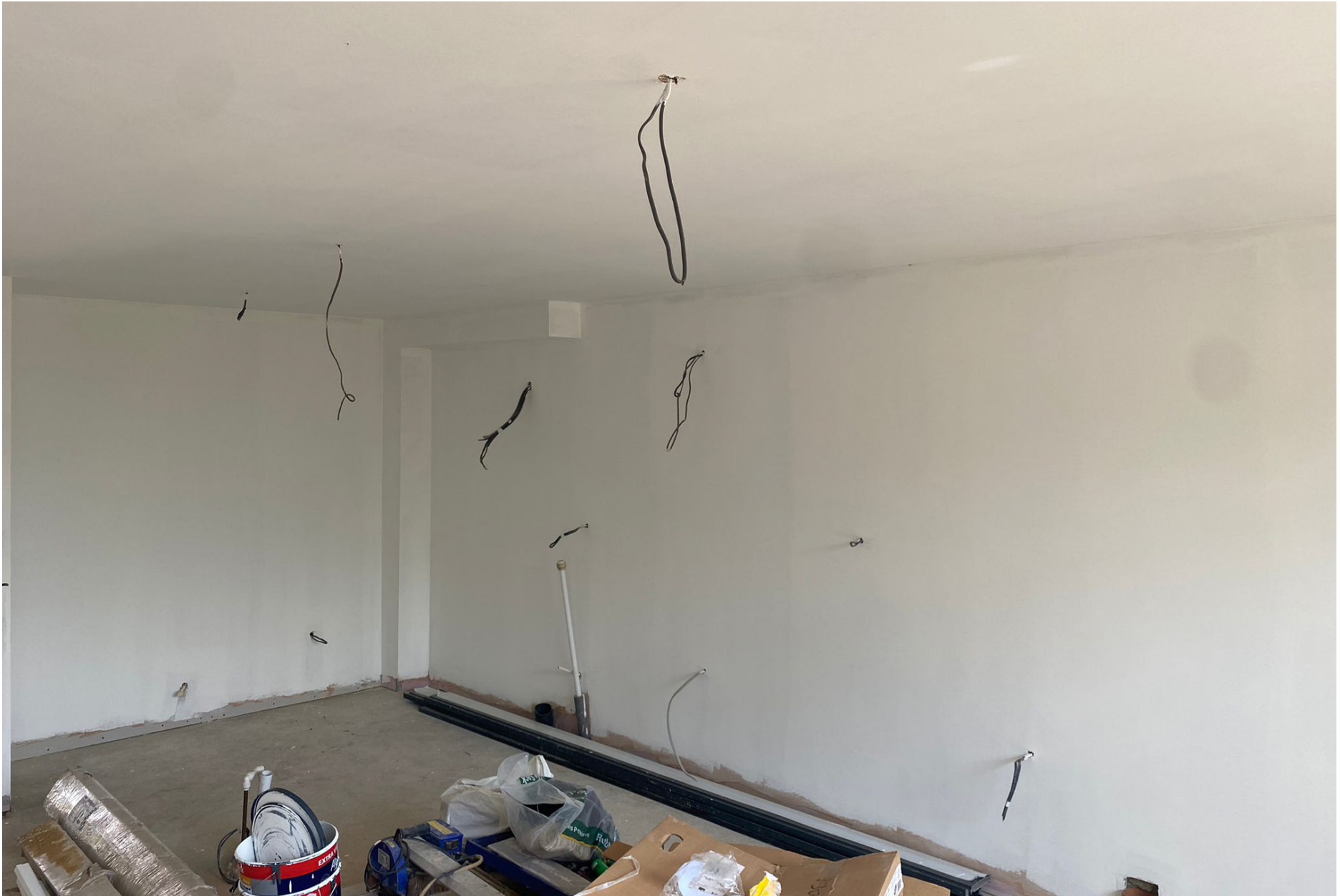
First fix electrics and plumbing have been finished ready for the arrival of the kitchen units.
